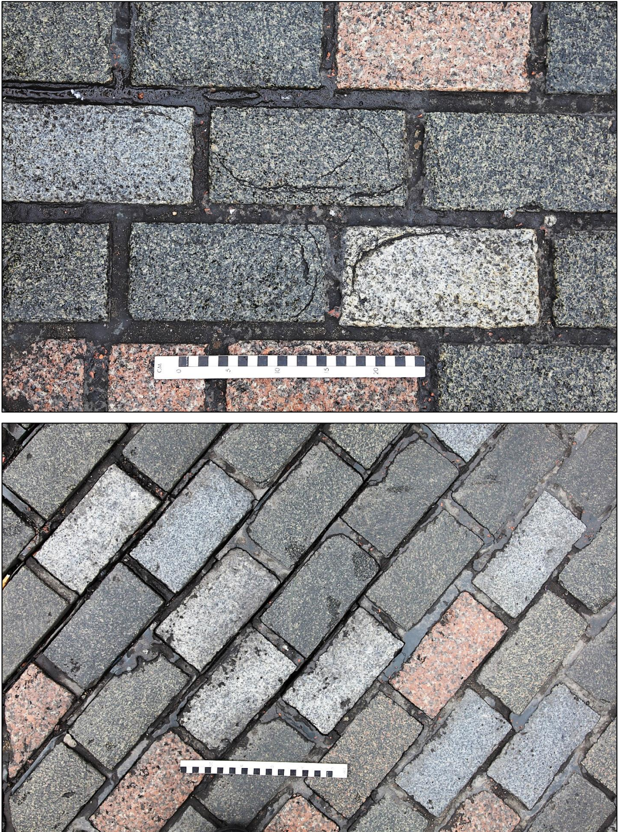
Figure 8 Performance issues in a recently setted area at the junction of South Bridge / North Bridge and Royal Mile
